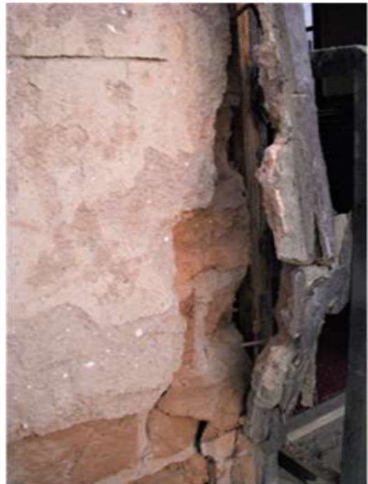
Figure 36: Basal wall damage to front of the church, Spring 2011. (Courtesy of Faith Hutson).
