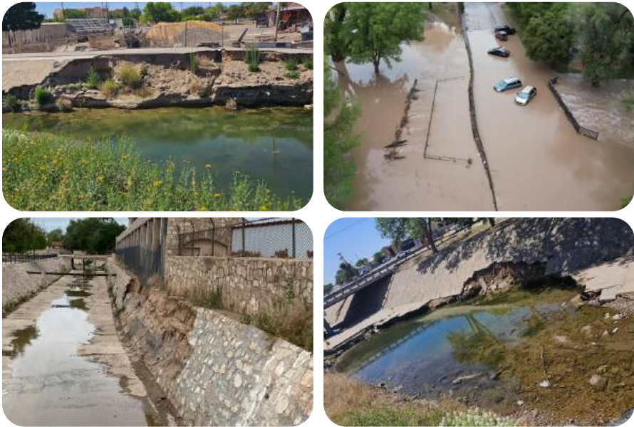
Figure 6.1 (A,B,C,D): Storm 2024 flooding and subsequent damages, Roswell, New Mexico
