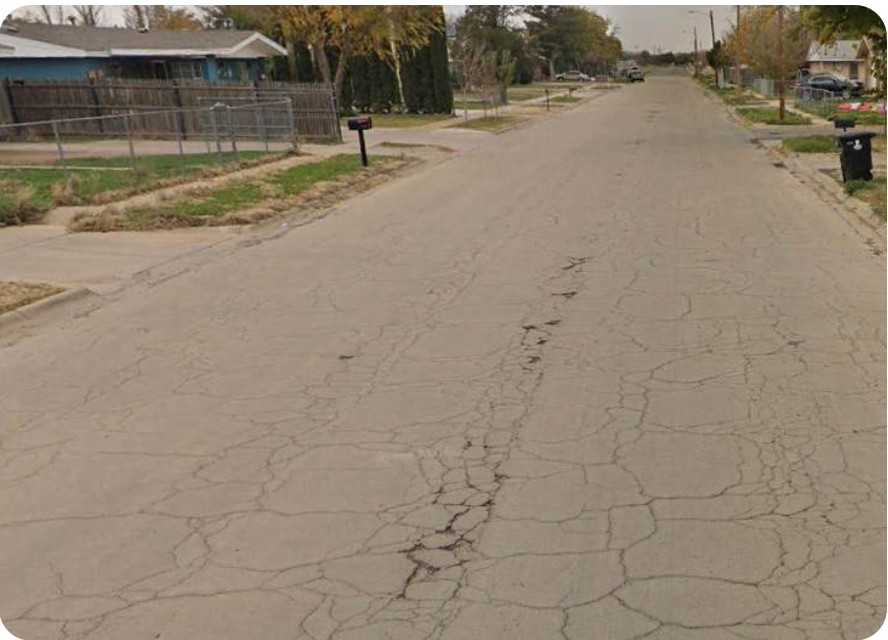
Figure 6.8: W. Jaffa Street Pavement Deterioration
