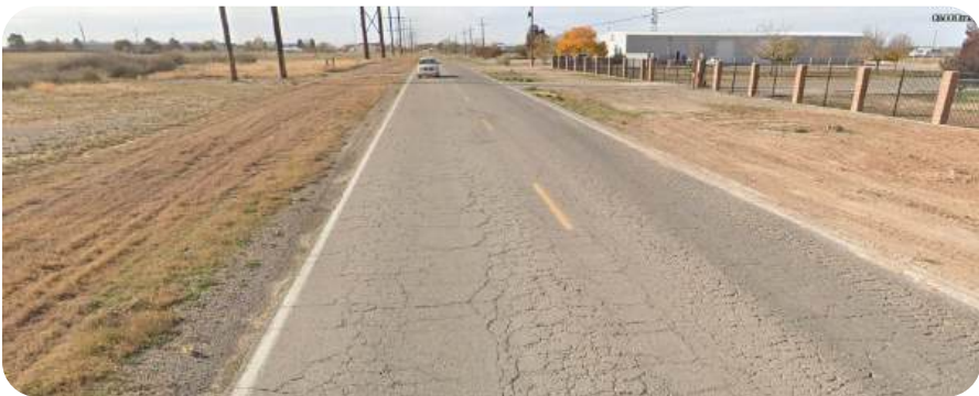
Figure 6.18 (A,B): Asphalt pavement distress at the intersection of W. Deming Street and S. Kentucky Avenue; Pavement failure/fatigue on E. Brasher Road
