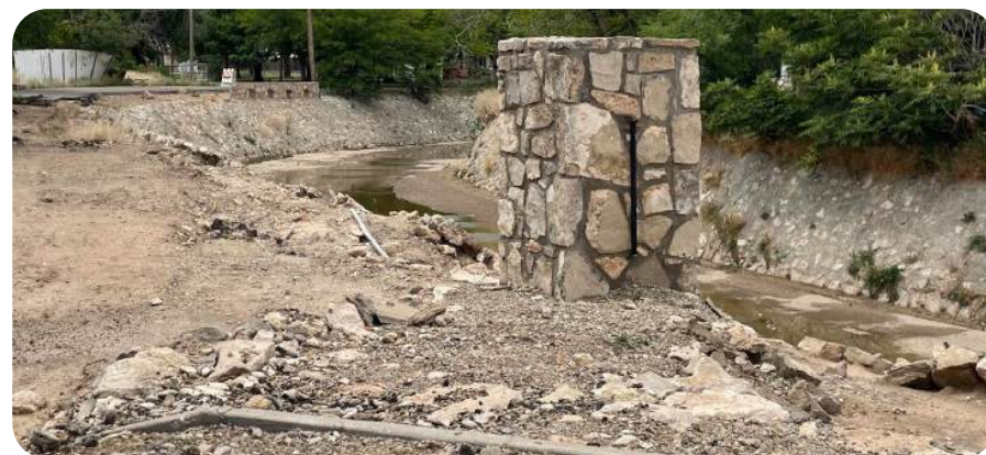
Figure 8.2 (A,B): Infrastructure Damaged by Flood
